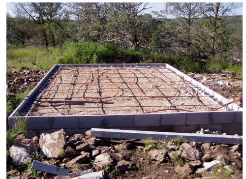
The nearly completed slab foundation for the Morgan telescope at Dark Ridge Observatory.
