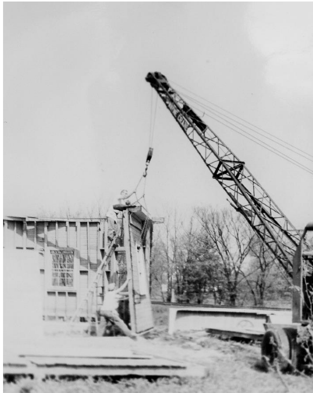
The work of re-assembling the observatory walls, mounting the telescope on the new pier, placing the dome in position and rebuilding the sliding shutters was all done by Ray Ulm, contractor, with his two assistants, Bob Miller and Paul Grilliot. The use of the large crane and its operator was donated by the Fruehauf Trailer Company. April-May- June 1960
